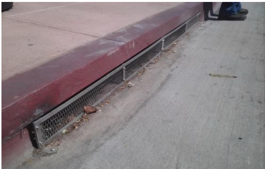
Internal Curb Inlet Debris Screen
