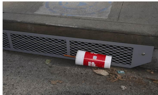
External Curb Inlet Debris Screen
