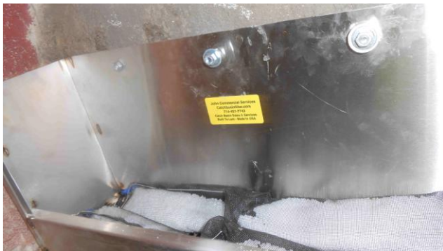
No Geo Cloth Bag To Clog Drainage
